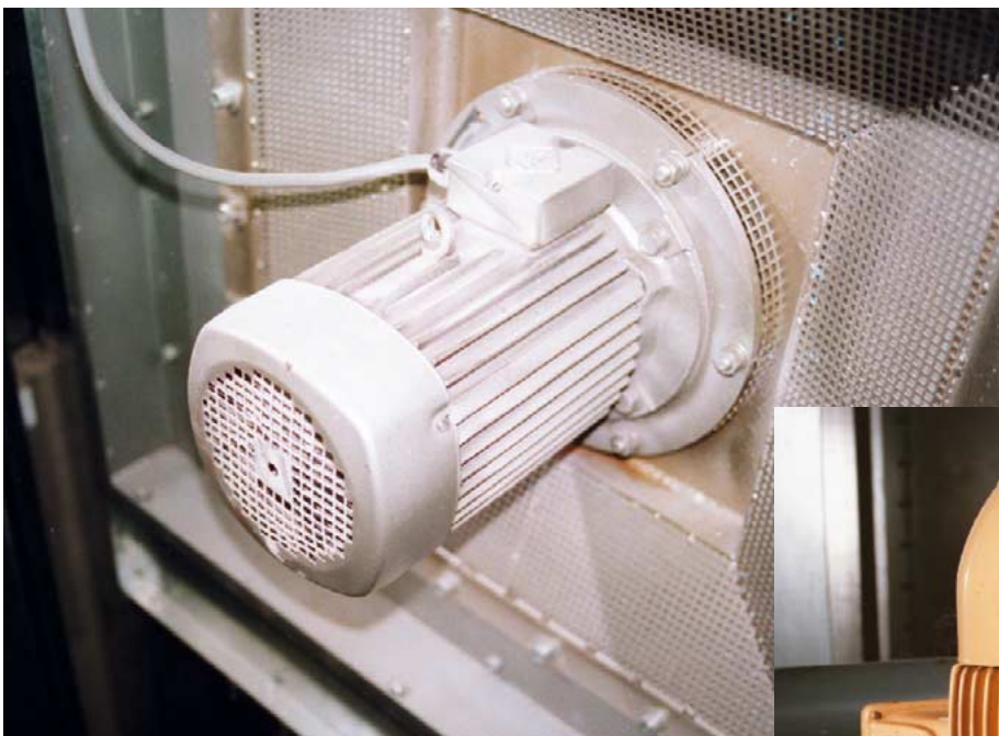
Monitoring a motor in a cooling system
